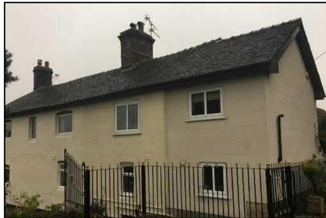
Inconsistent facade treatments
