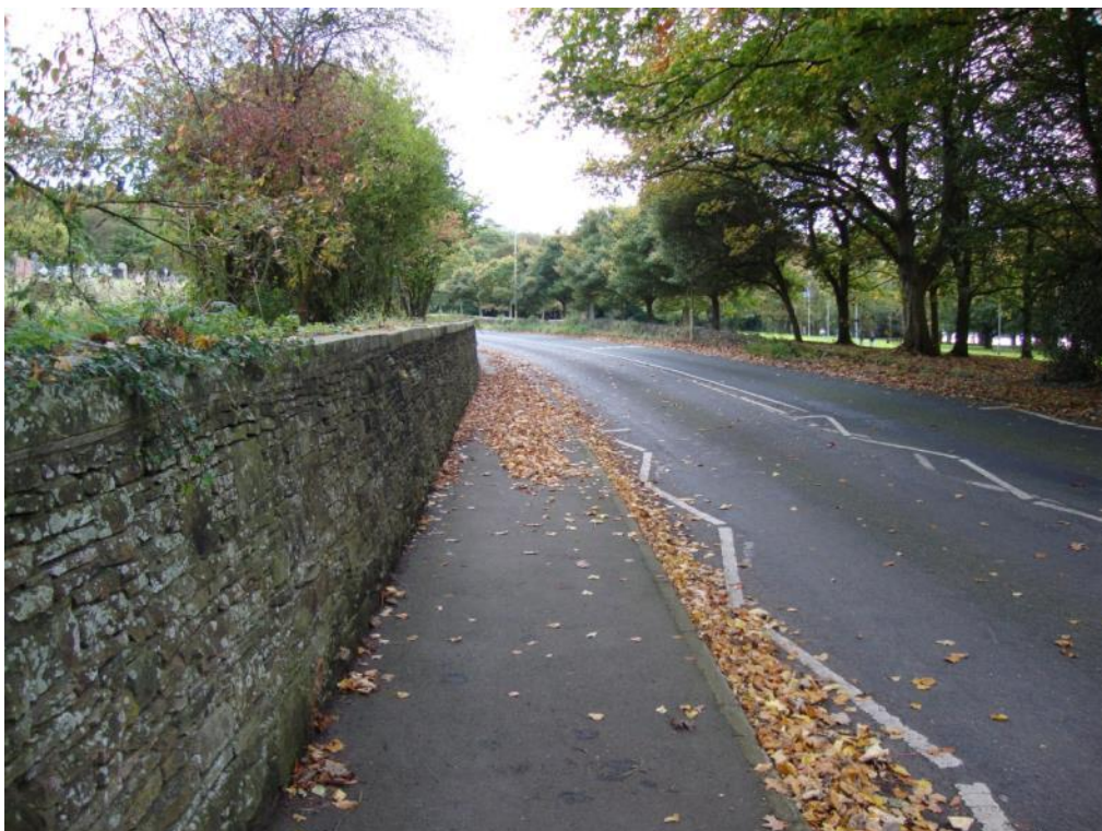
Above: The sandstone wall on the perimeter of the churchyard of the Church of St John the Baptist.
